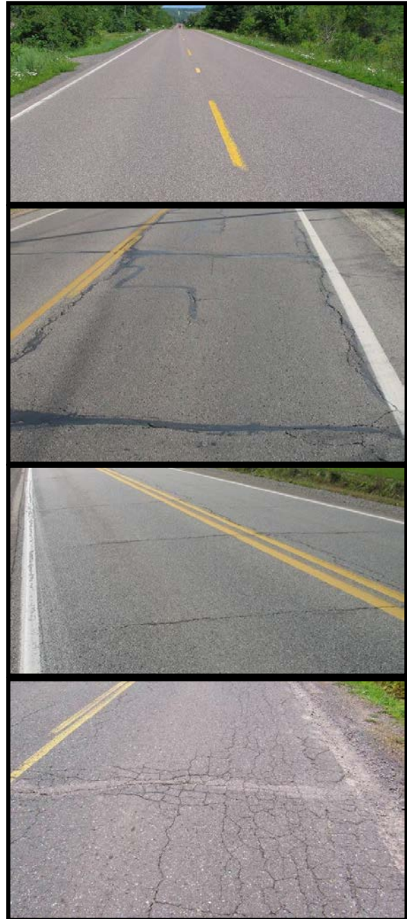
Figure 1: Top image, right –PASER 8 road that is considered “good” by the TAMC exhibit only minor defects. Second image –PASER 5 road that is considered “fair” by the TAMC. Exhibiting structural soundness but could benefit from CPM. Third image – PASER 6 road that is considered “fair” by the TAMC. Bottom image – PASER 2 road that is considered “poor” by the TAMC exhibiting significant structural distress.
